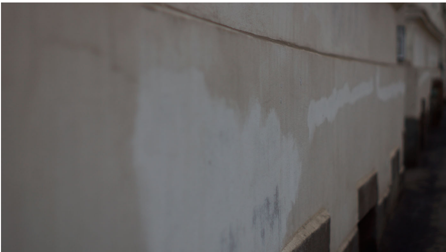
Figure 6 Painted-over graffiti, creating a negated space along a wall (2017)
